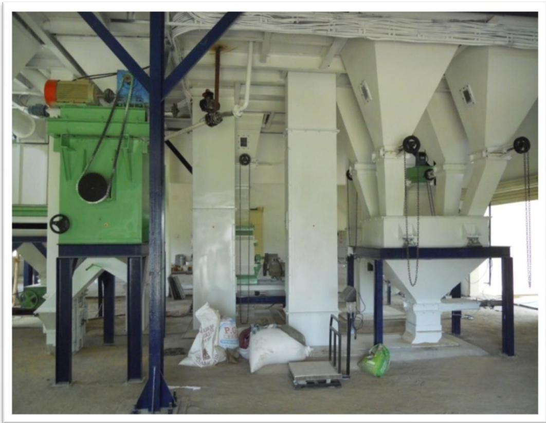
FEED PROCESSING EQUIPMENTS
